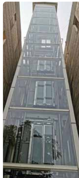
Actual Site Image of Structure lift with Glass Installed in Parwana Apartments Delhi
