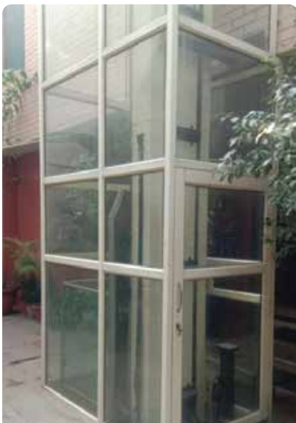
Actual Site Image of HEXA Hydraulic Lift
